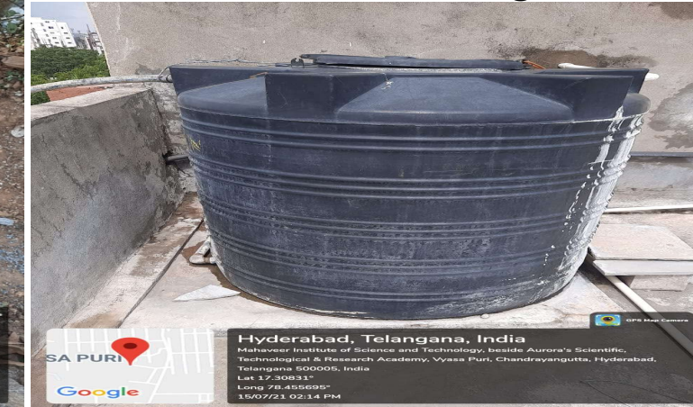
Overhead Water Storage Tank
